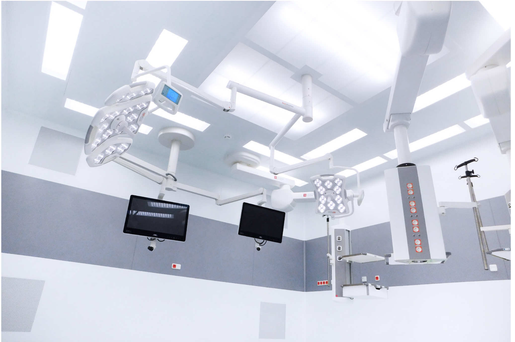
Annex Building of the 5th Operating Theatre and Connecting Links, Hospital Hořovice | Czech Republic | 2018
