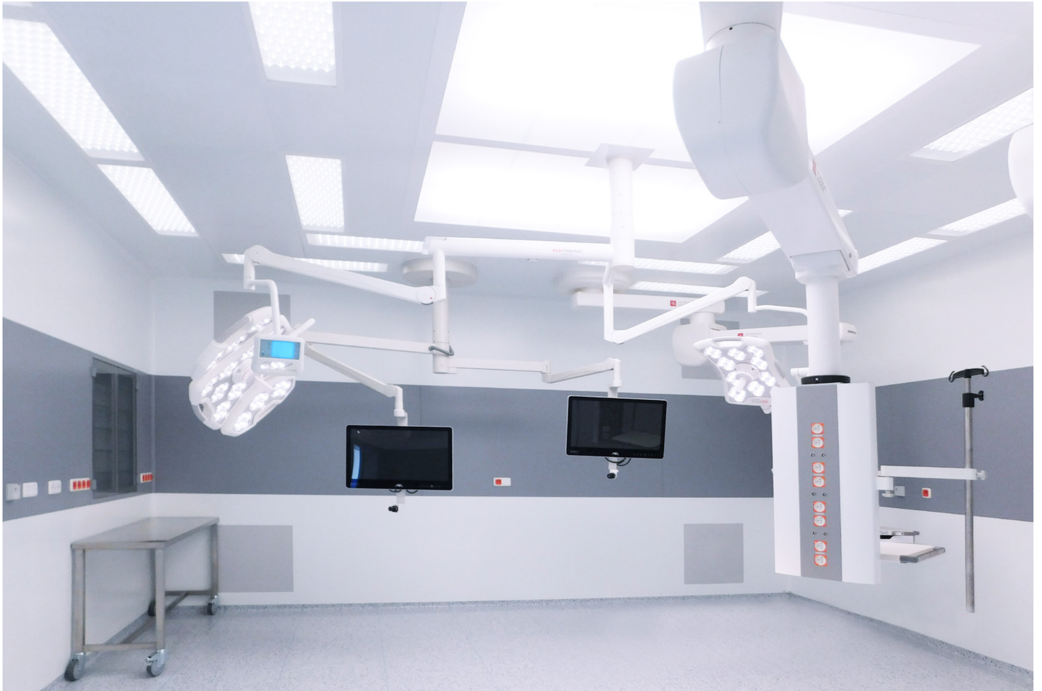
Annex Building of the 5th Operating Theatre and Connecting Links, Hospital Hořovice | Czech Republic | 2018
