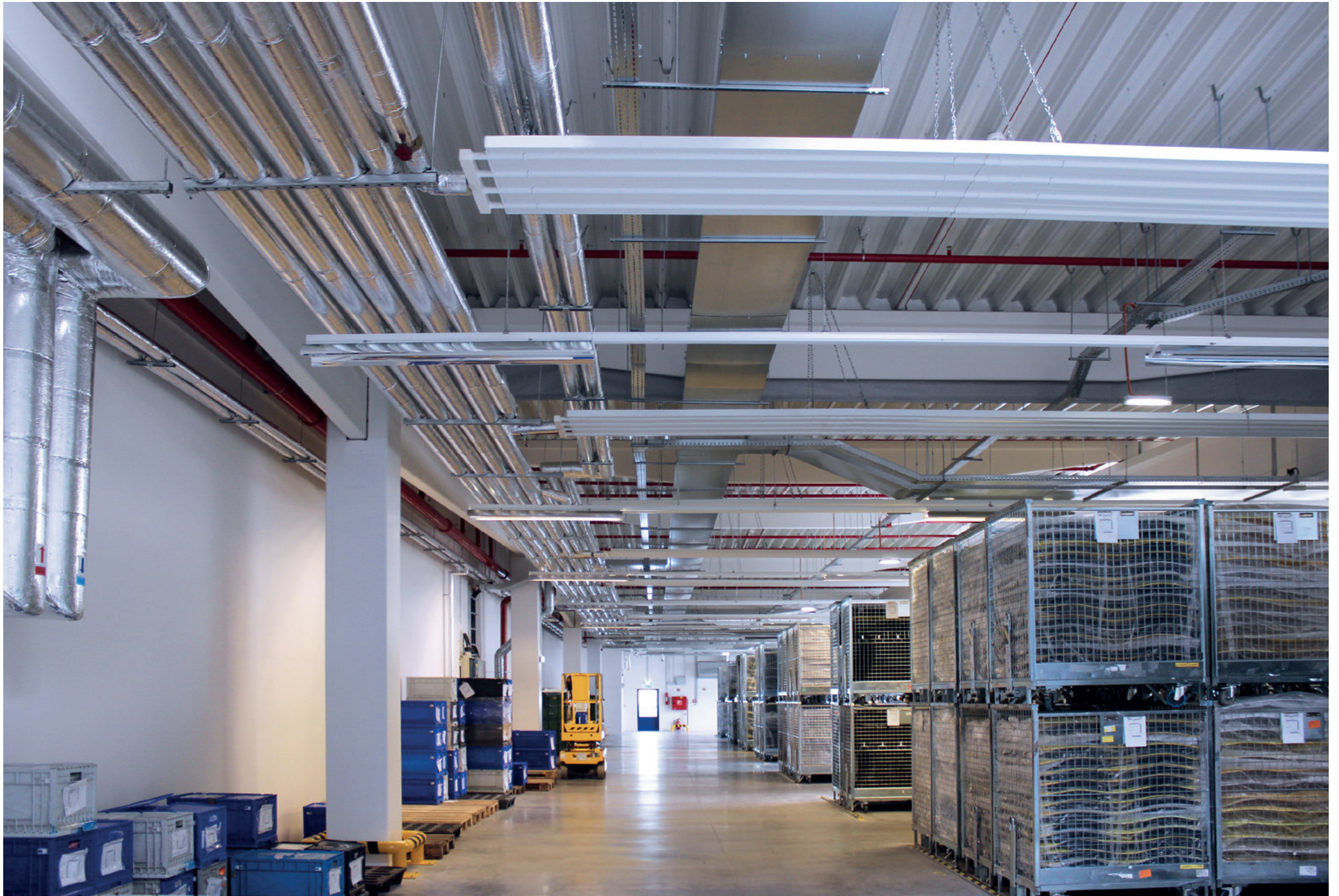
Ventilation of the assembly hall B10 in the plant HAT Mohelnice; HELLA; Mohelnice; Czech Republic; 2012
