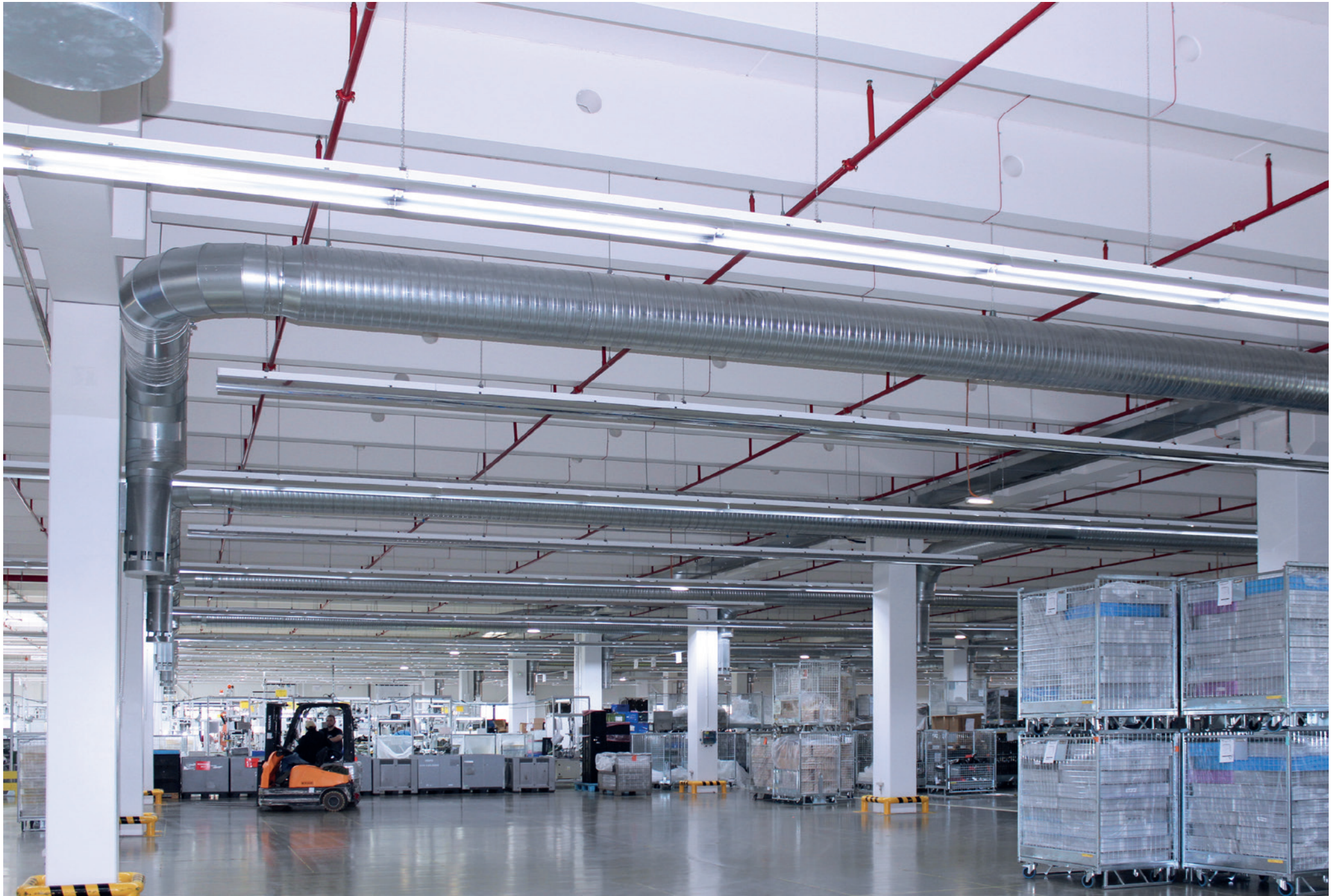
Ventilation of the assembly hall B10 in the plant HAT Mohelnice; HELLA; Mohelnice; Czech Republic; 2012
