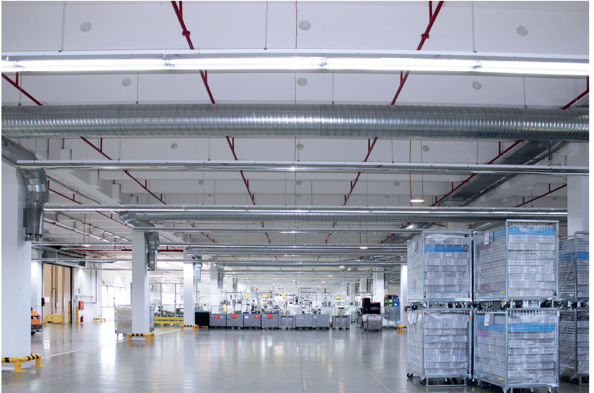
Ventilation of the assembly hall B10 in the plant HAT Mohelnice; HELLA; Mohelnice; Czech Republic; 2012
