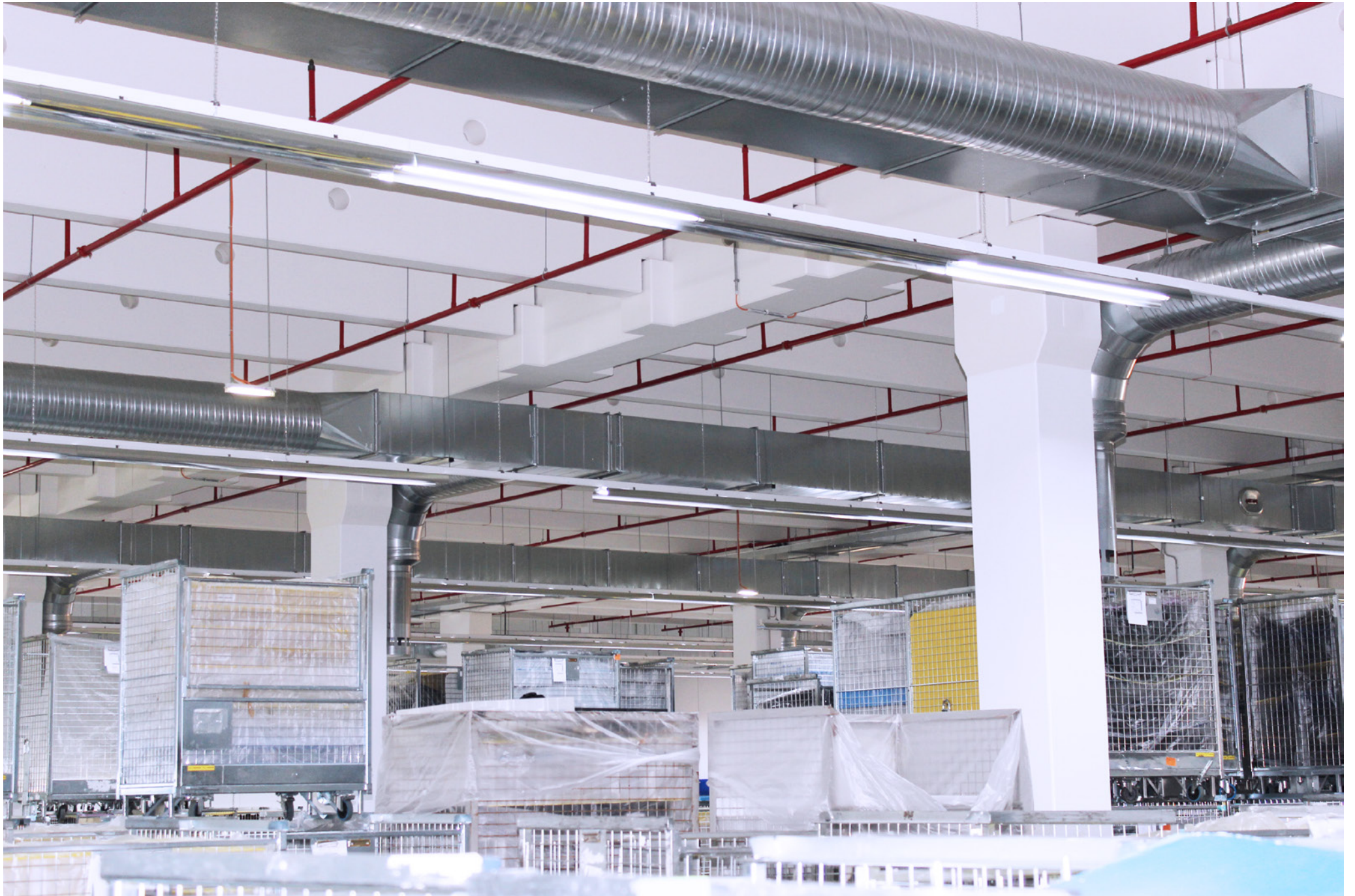
Ventilation of the assembly hall B10 in the plant HAT Mohelnice; HELLA; Mohelnice; Czech Republic; 2012
